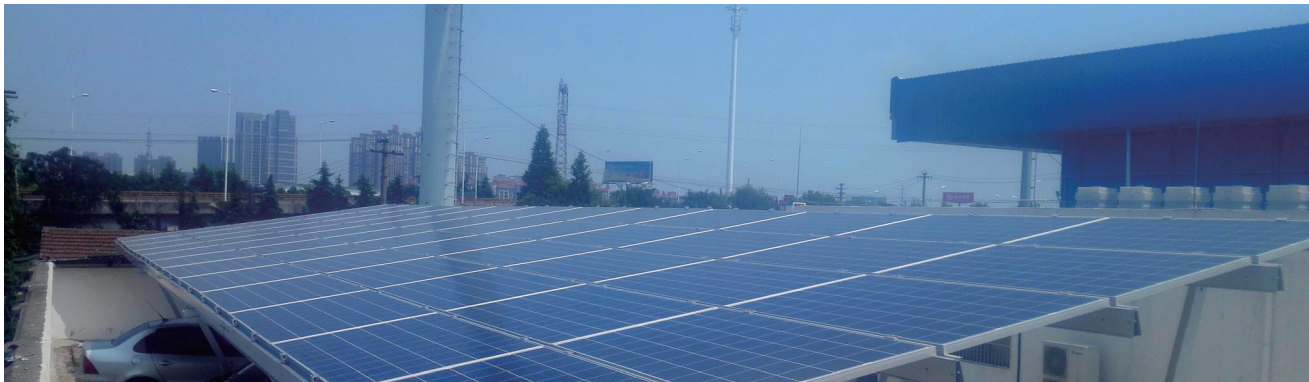
Sinochem-Total Solar-Powered Gas Station Project Location: Wuxi, Jiangsu PV Capacity: A total of 120 PV modules were installed, with an installed capacity of 30 kW; annual electricity generation is projected to reach 35,370 kWh. Model: Self-generation for self-consumption.
