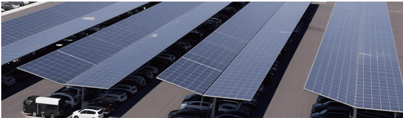
Lebanon Carport Location: Matn District, Lebanon PV Capacity: 250 kW PV system, comprising 240 pieces Tiger Neo 3.0 modules , Energy Storage Capacity: 3.34 MWh Model: Self-generation for self-consumption
