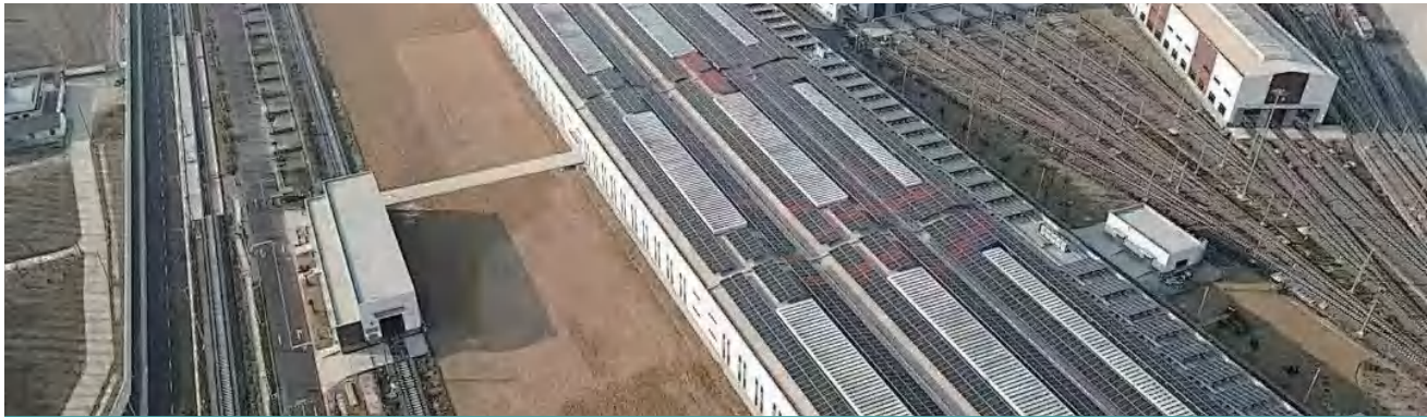
Shanghai Metro Line 14 6.56 MW Project Location: Fengbin Base, Shanghai PV Capacity: 6.56 MWp PV system, capable of generating approximately 6.7 million kWh of green electricity in the first year of operation. Model: Self-generation for self-consumption
